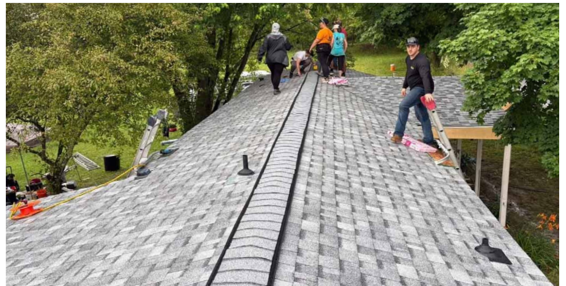
Courtesy photo A roof is replaced on a home in Masontown by volunteers during the 2025 Summer Home Repair Program.
