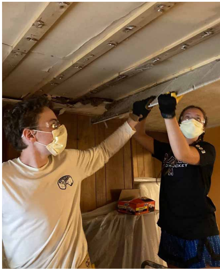
Courtesy photo Two volunteers fix a ceiling in a Newburg home during the 2025 Summer Home Repair Program.
