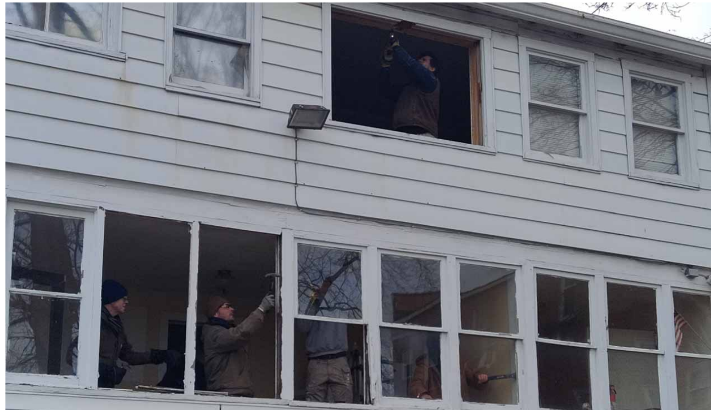
Dom Pileggi, top, John Guiney and Aidan Pressl prepare the frames for new windows to be installed Jan. 24 at the building recently purchased on West King Street in Martinsburg by Mary's Refuge.
