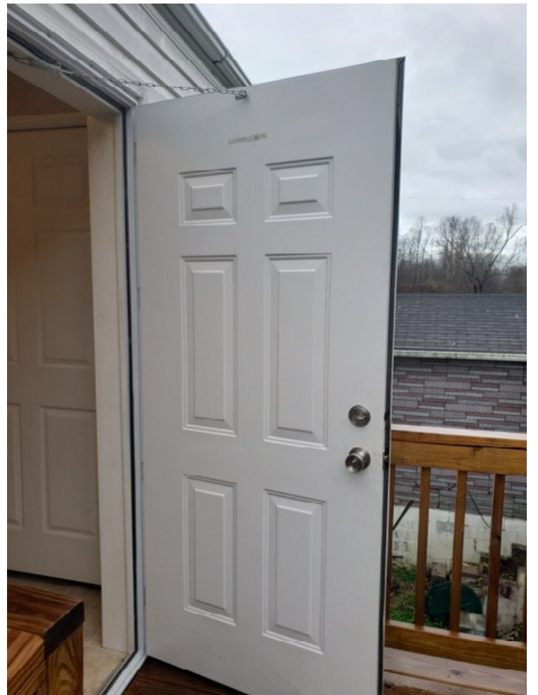
Courtesy Photo Catholic Charities West Virginia's Disaster Services program installed a new door for a rebuilt home of a flood survivor.
