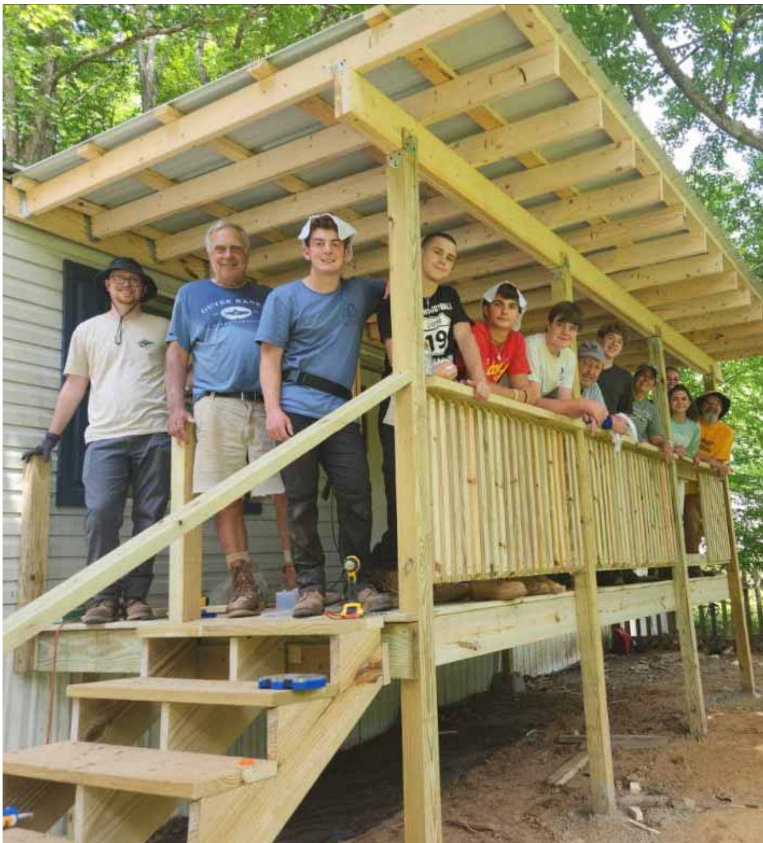
Courtesy photo Volunteers for the Summer Home Repair Program in Preston County stand on the new back porch they built for an individual in need.
